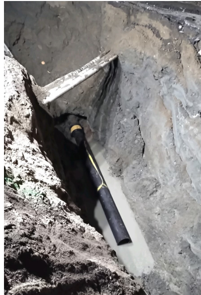
Left: Sewer main break on Barrett Road near Pearl Street. The excavated area is pictured before the installation of a trench box that is designed to protect the workers in the trench.
